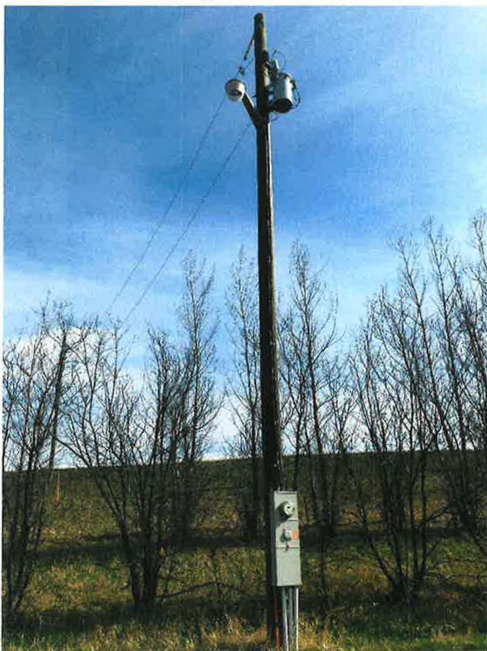
Photo 19: Power pole with transformer present south of the garage near the residential home on Site.
