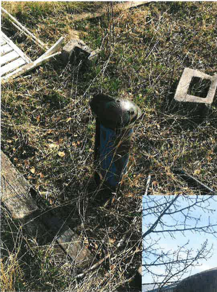
Photo 21: Water supply well located to the east of the mobile home and garages. Wires to connect a pump were still present in the well
