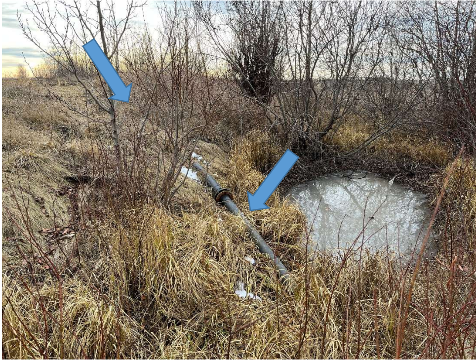
31. Close up view of the pipeline (arrows) leading from the pump house on the Olds Golf Course property; photograph taken facing southwest.
