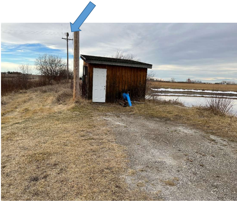
29. Pump house and pole-mounted transformer located on the Olds Gold Course property; photograph taken facing west.
