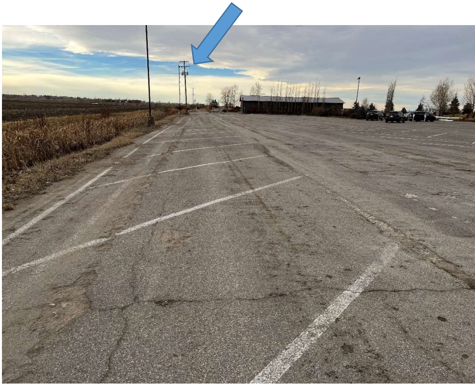
25. View of the pole-mounted transformers (arrow) located on the Olds Golf Course property; (arrow); photograph taken facing west.
