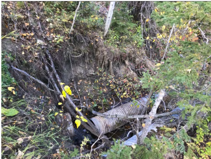
Damaged culvert causing slope failures
