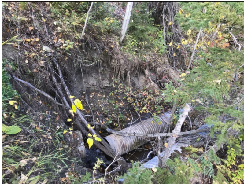
Damaged culvert causing slope failures
