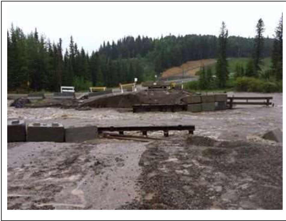
RR 5.2 TEMPERARY BRIDGE LOCATION NORTH OF WATER VALLEY TAKEN THURSDAY JUNE 20 TH , 2013
