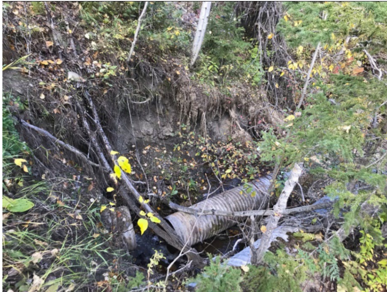
Damaged culvert causing slope failures
