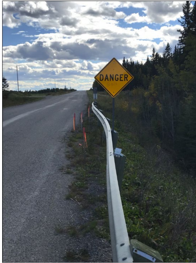
Damage to road and guardrail caused by slope failure.
